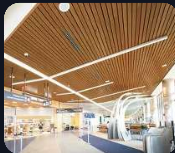
Airports & metro stations
